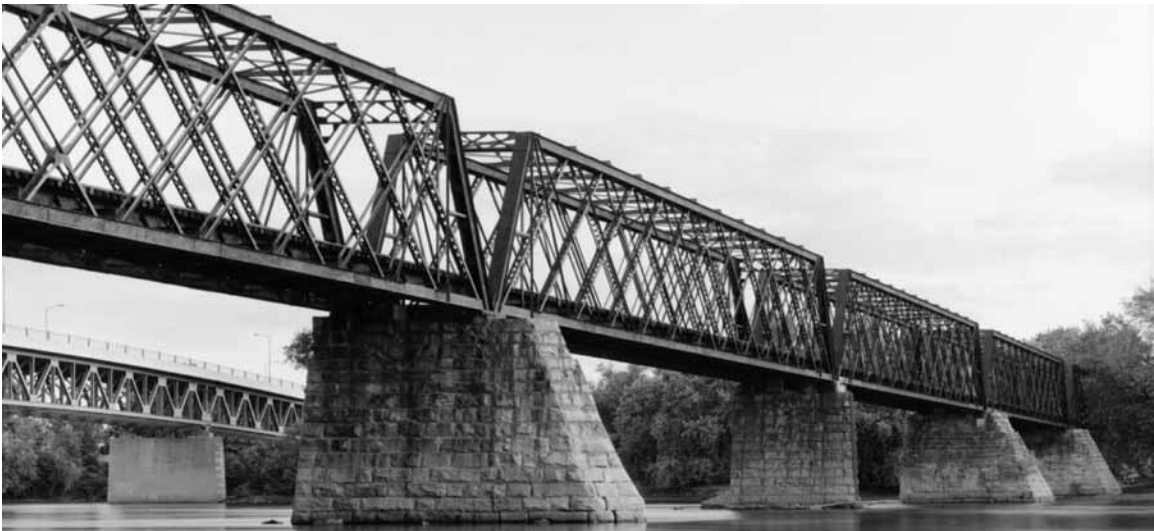
14. Boston & Maine Railroad Bridge, with State Route 9 highway bridge in background, Northampton, MA
